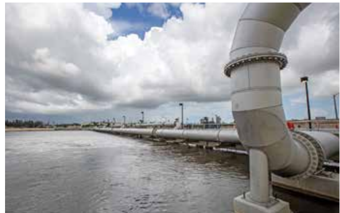
Piping carries air to one of the facility's aeration basins, which are outfitted for biological nutrient removal.
