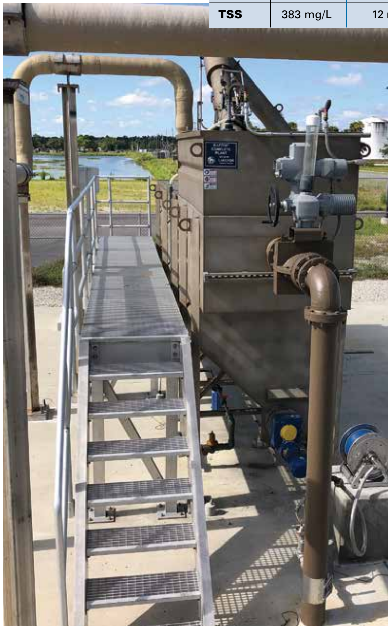
Septage and FOG are accepted at the Raptor receiving station (Lakeside) and co-digested to produce biogas.
